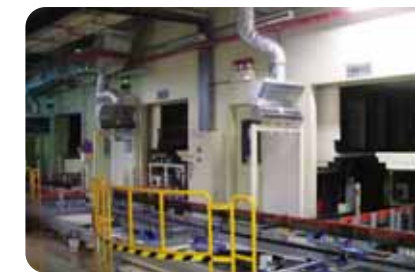
PDP Manufacturing Process Exhaust System in Cheonan Plant
